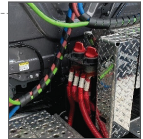
Figure 13. Driver-side battery disconnects
