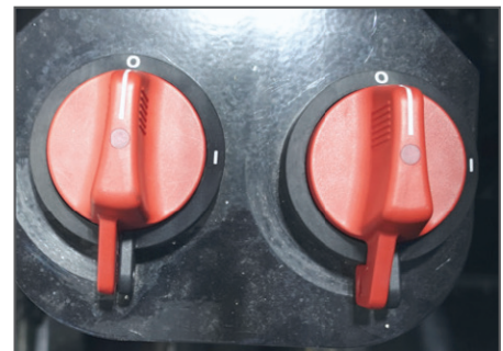
Figure 10. Switches in off position
