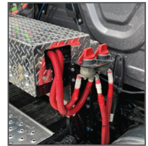
Figure 12. Passenger-side battery disconnects
